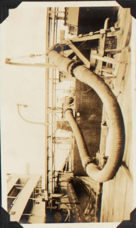
SS. VOCCO PUMPING MOTOR SPIRIT THROUGH A 10 INCH LEAD. RATE OVER 100,000 GALLS. PER HOUR.
