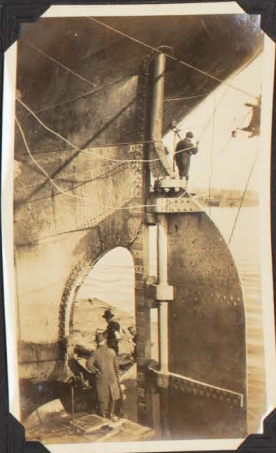
REPAIRS WHILE YOU WAIT, REPLACING PROPELLAR BLADE LOST AT SEA. SS "CANADIAN SEICNEUR" PRINCES WHARF.
